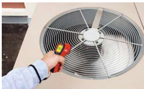
Measure efficiency of heat dissipation to reveal and locate thermal losses in the flow system.
