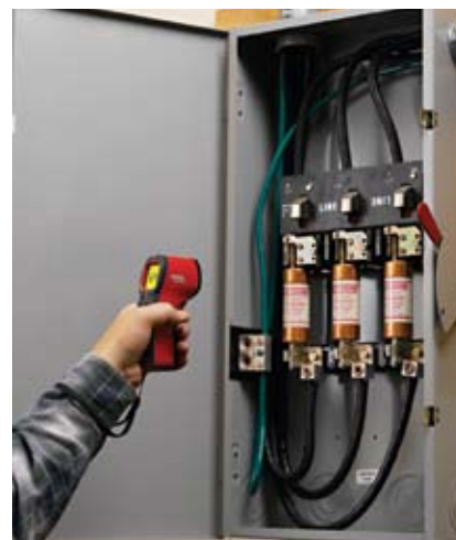
Check fuse or circuit breaker overheating, which could be caused by overloaded circuits.
